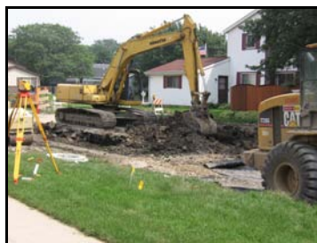
Picture of an Undercut of Residential Street
